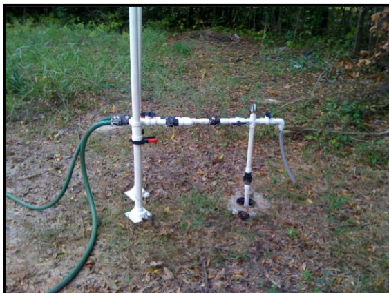
Multi – Phase Injection Manifold
